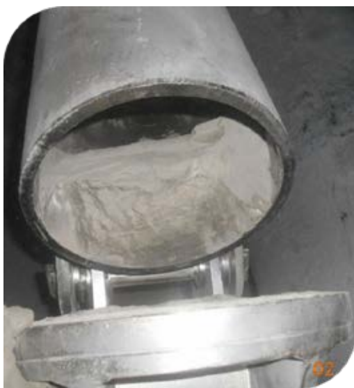
Figure 4 - Formation of coke inside the cyclone's dip leg. Source: FCCSA's archives.
