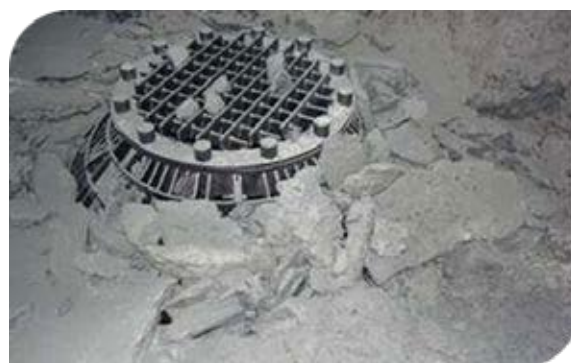
Figure 5 - Coke that detached from the reactor walls causing partial obstruction of the catalyst outlet. Source: FCCSA's archives
