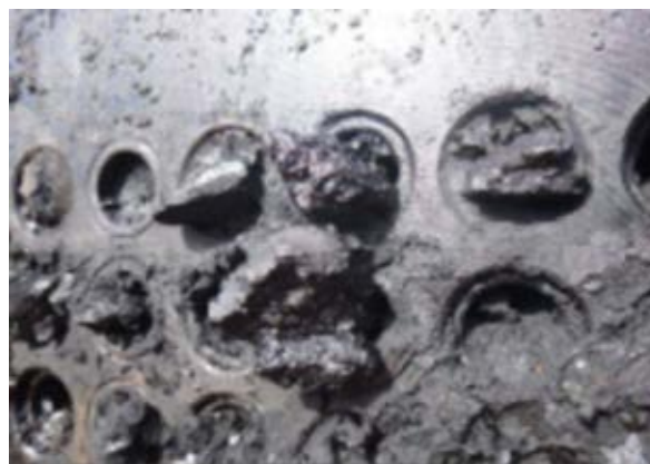
Figure 11 - Heat exchanger blockage by coke. Source: FCCSA's archives
